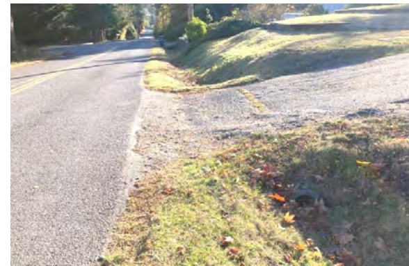
Existing stormwater drainage ditches in the ROW could be retrofitted to provide water quality treatment and infiltration.
